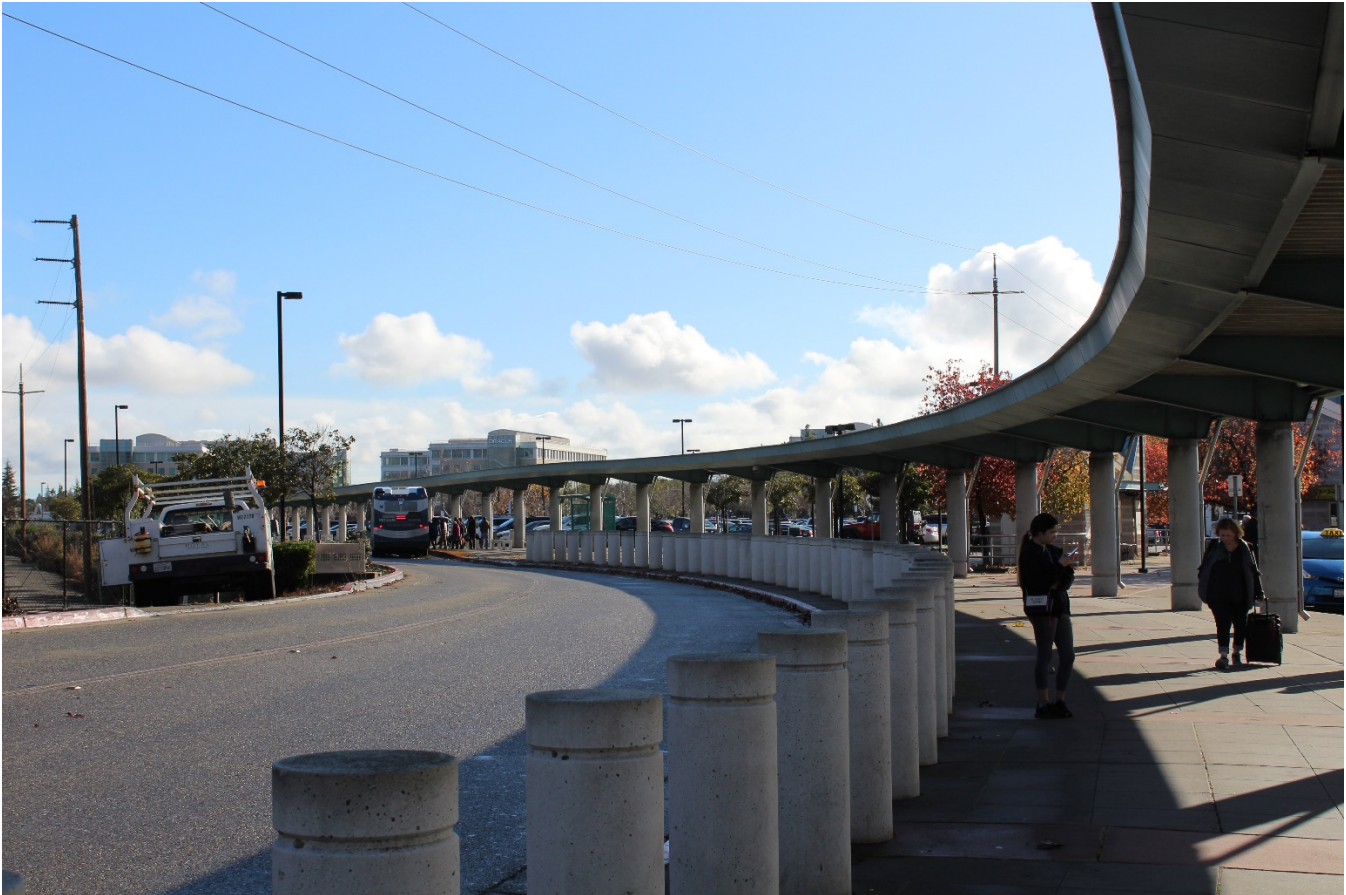
Figure 42. Overhead Cover Pleasanton Side of Station
